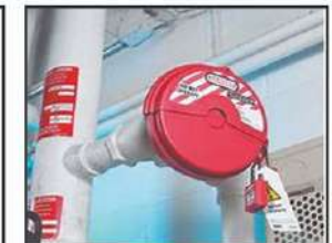
127. Gate Valve Lockout
