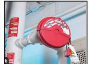
127. Gate Valve Lockout
